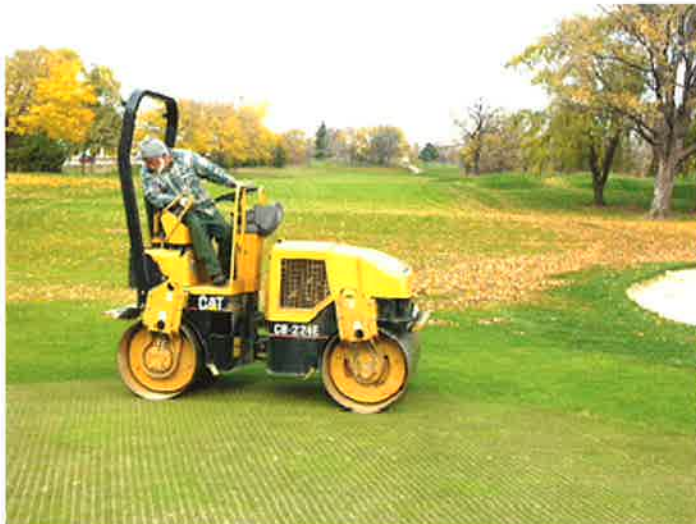
A heavy roller can help restore surface drainage through the perimeter of the greens by lowering the grade of an elevated collar.
